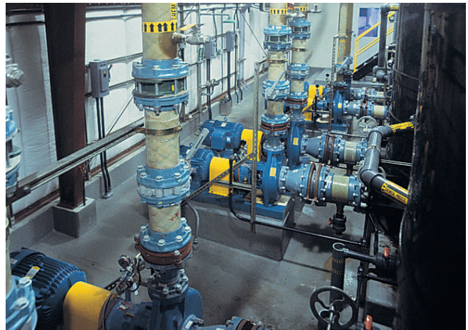
Multi-stage scrubber pump room.
