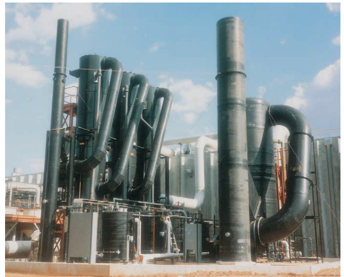
Tri-NO x Multi-Chem plant constructed of black, UV-stabilized polypropylene with external recirculation systems and catwalk access assembly.
