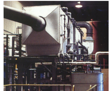
Multi-stage horizontal NO x scrubber applied to steel pickling line.
