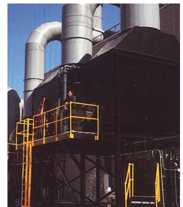
A 60,000 CFM AnoVent system venting a bright dip operation.
