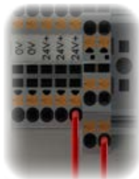
CONNECTION FOR CLEAN AIR VF (USE PROXIMITY SENSOR CONNECTIONS, JUMPER IF NOT USED)
